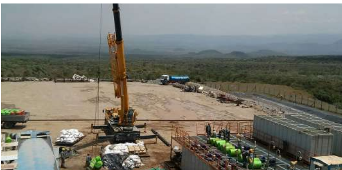
AKIIRA GEOTHERMAL POWER PLANT | Kenya
