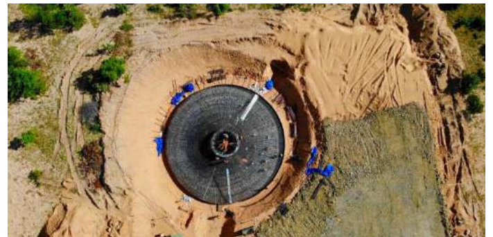
DAI PHONG WIND FARM | Vietnam
